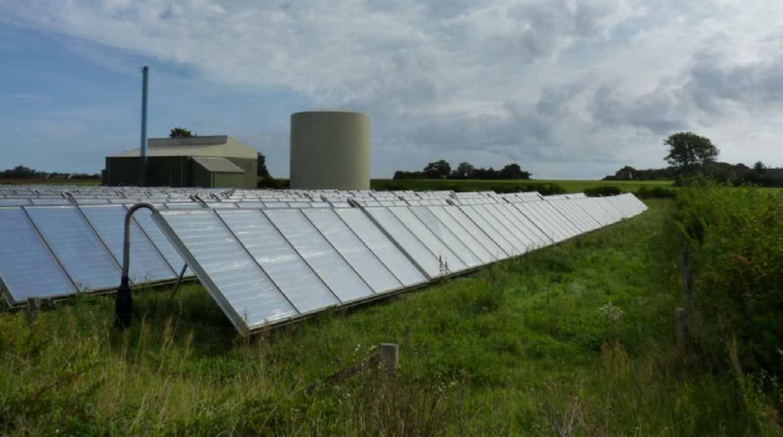
Figure 8: solar boiler field and district heating plant at Nordby, Samsø (copyright Sven Stremke).
